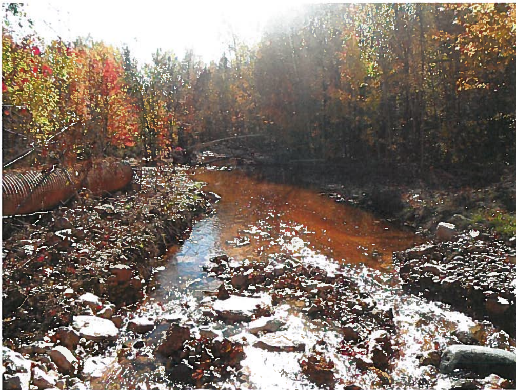
Photographs 19 and 20. Examples of the catastrophic failure of a beaver dam, with bottom photograph showing a road and culvert that were washed out following failure of dam (October 9, 2013).
